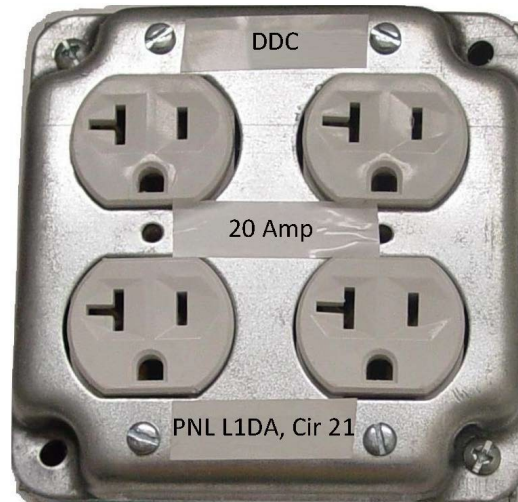
Figure 2-10. Dedicated Outlet Labels – Example
